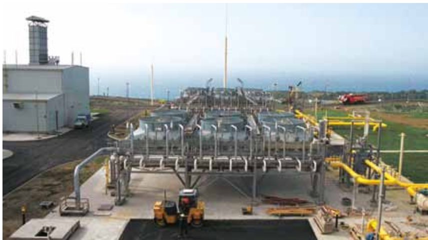
Beregovaya compressor station – starting point of Blue Stream
