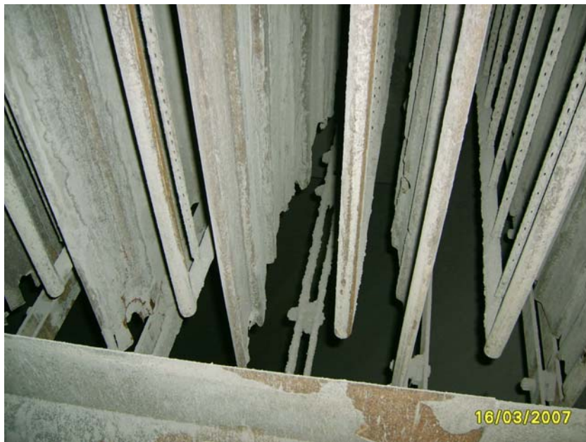
Electric filters in boiler 5 at Troitsk SDPS in 2007
